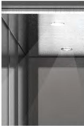
Aluminium Ceiling & LED lighting
